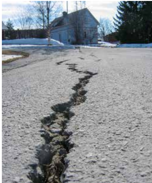
Earth quake damage on a road.
